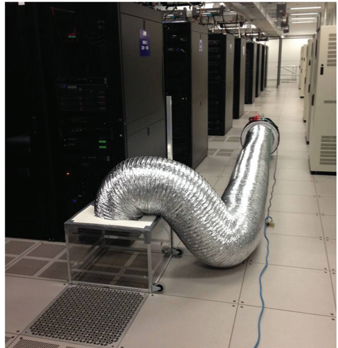
Figure 5 Powered flow hood (PFH).
